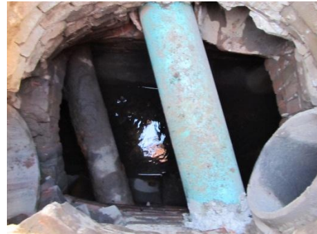
Man hole on Woodward Ave where sewage observed to be dumping into the storm drain (Top). The Woodward Ave manhole after the broken and leaking pipes were replaced (Bottom).
