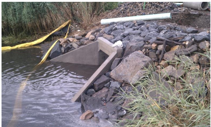
Moody's Lane storm drain discharge before (Top) and after (Bottom) construction to replace the storm sewer line.
