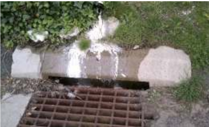
Pipe connected to 58 W Branchville Rd that drains into the storm drain. Photo taken on 5/7/12.
